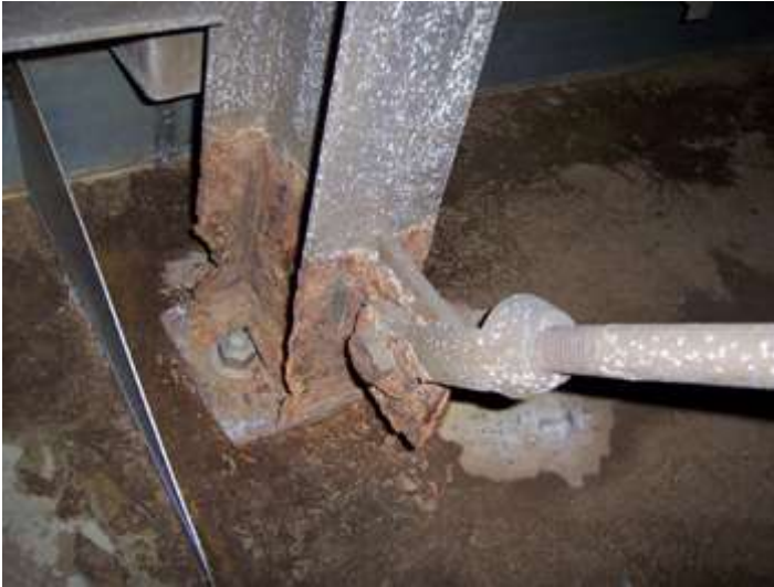
Photo #1: Existing rusted Aluminum column bases
