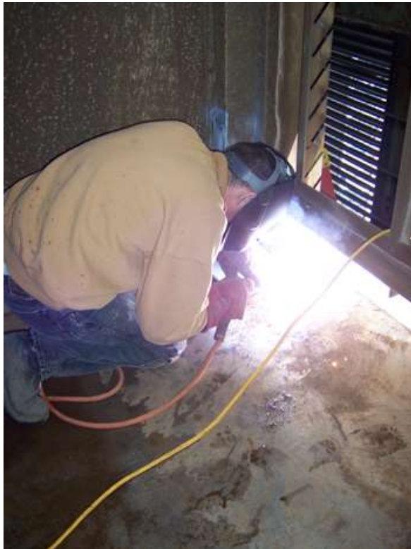
Photo #3&5: Welding new column bases view of the tower structure interior space
