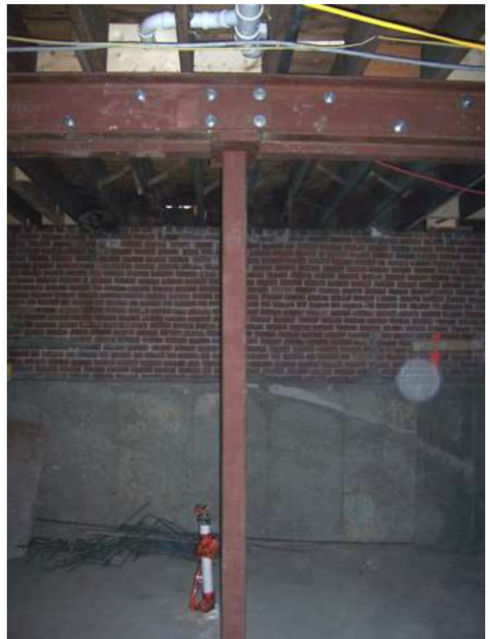
Photo #4: Existing roof beam was reinforced with new steel channels supported on new steel columns
