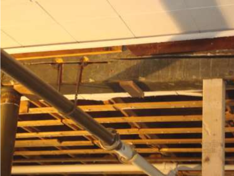
Photo #1: Existing cracked beam replaced
